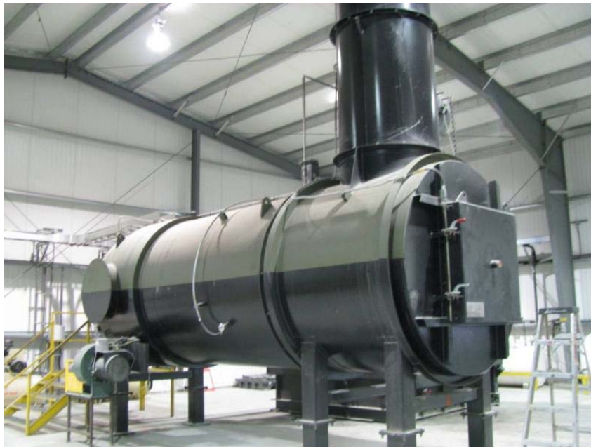
Photo 6: Dual chamber forced air incinerator.
