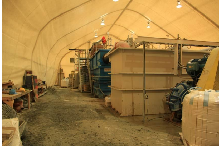
Photo 9: Water treatment facility
