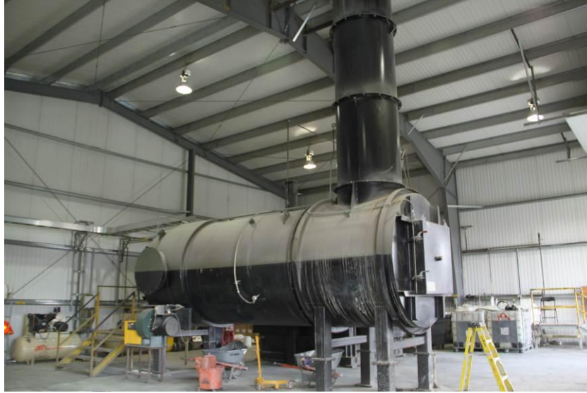
Photo 11: Dual chamber forced air incinerator at the Meadowbank site
