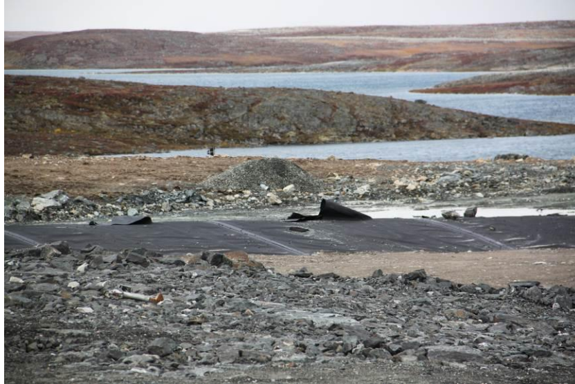
Photo 7: Ripped liner at Saddle Dam #1
