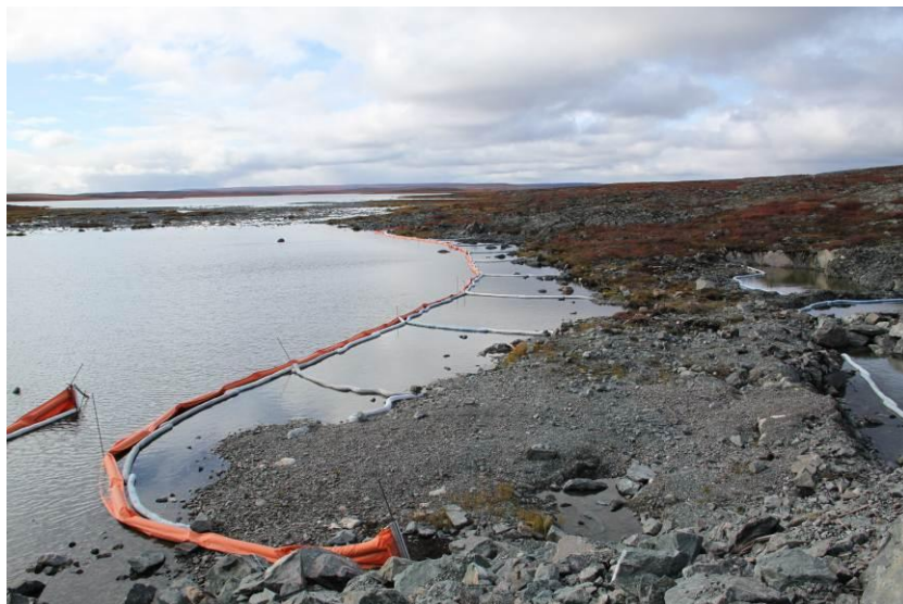
Photo 17: Booms and screens in place at HADD bridge to prevent any fuel from entering stream
